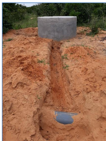
A slab for a proposed new water point at Mtsara wa Tsatu village undergoing curing
